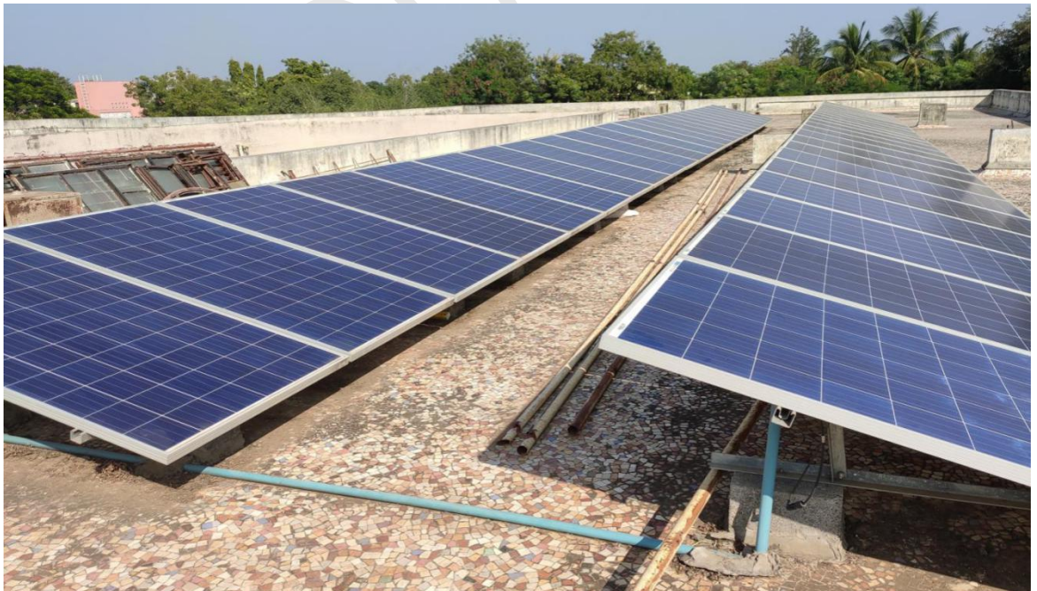
Solar On Grid (15kWp)
