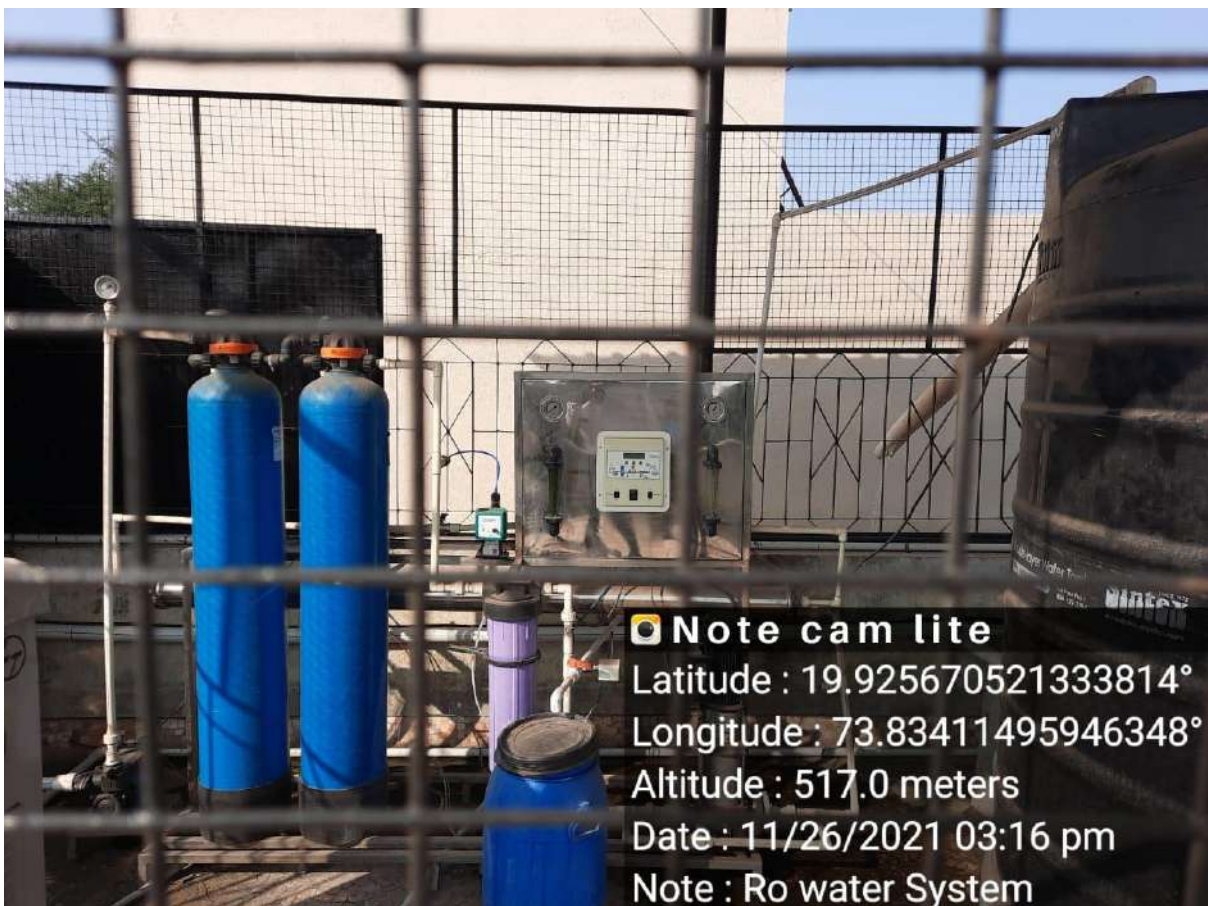
Figure.6. RO Water Purifier system
