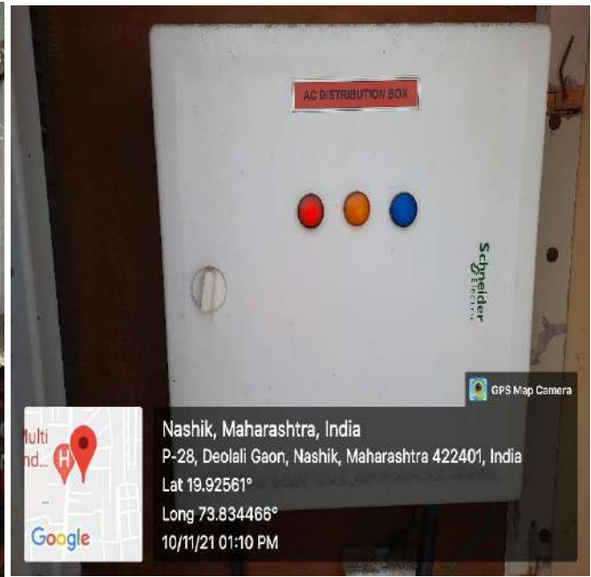
2. AC Distribution box
