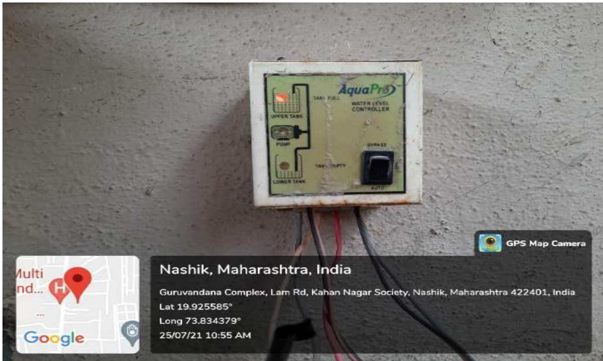
Sensor based energy conservation- Installed sensors for water pump and main water storage & distribution tank
