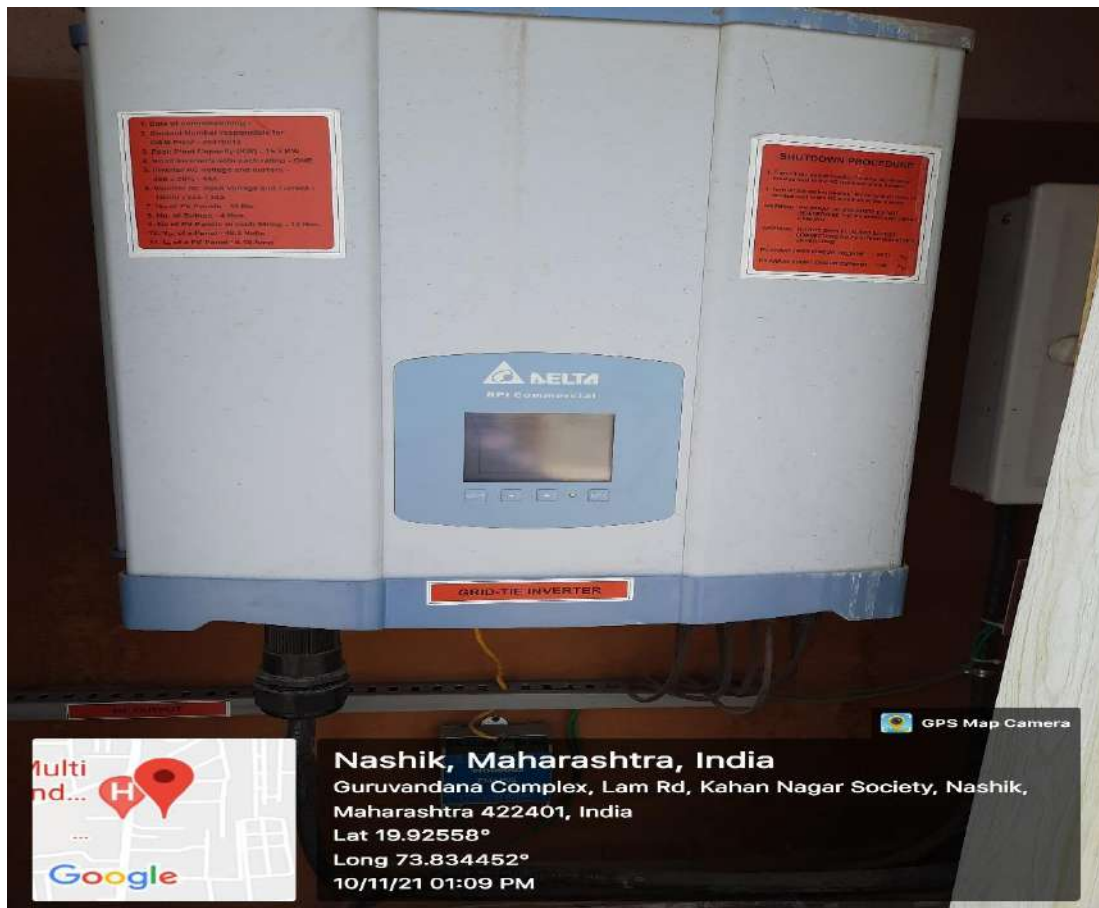
GRID- TIE INVERTER of Solar Panel
