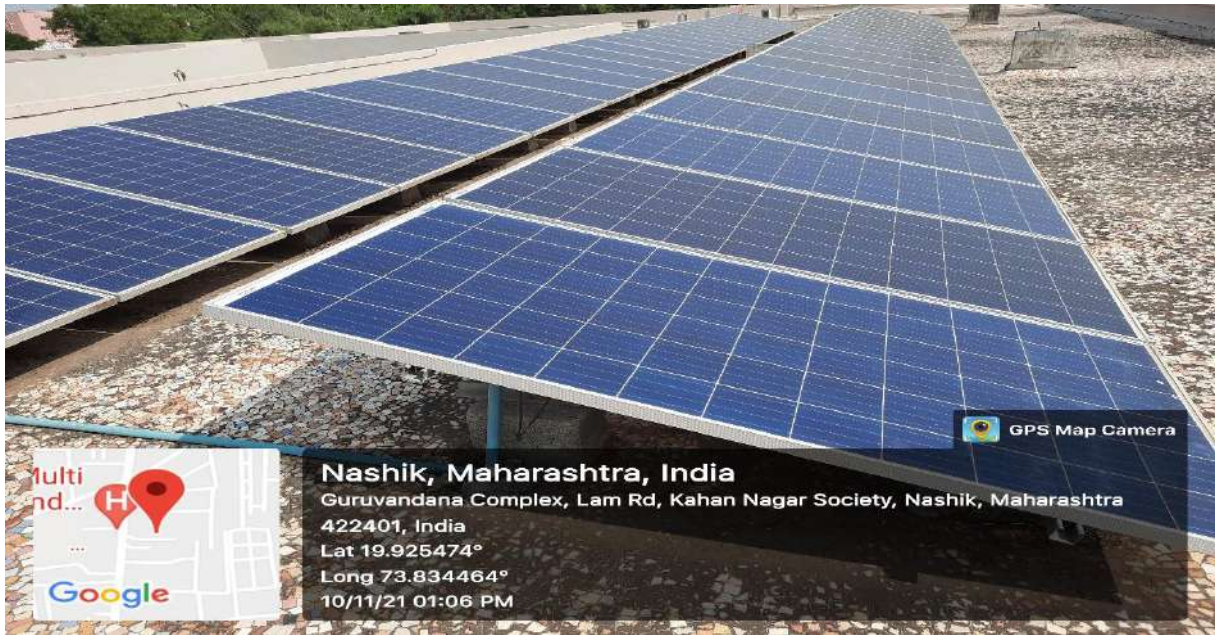
1. Solar Panel installed on Rooftop
