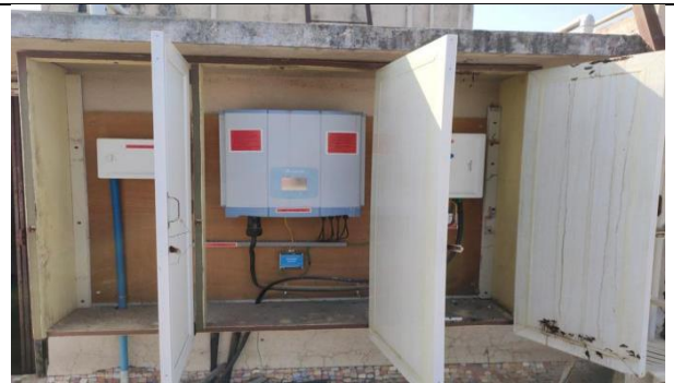
Grid tie Inverter 15.6 kw
