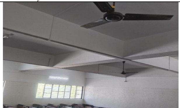
Class Room: showing fan & LED tube
