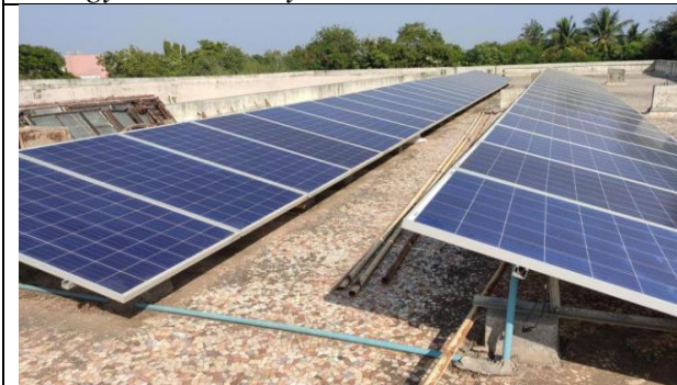
Roof Top Solar panel Array
